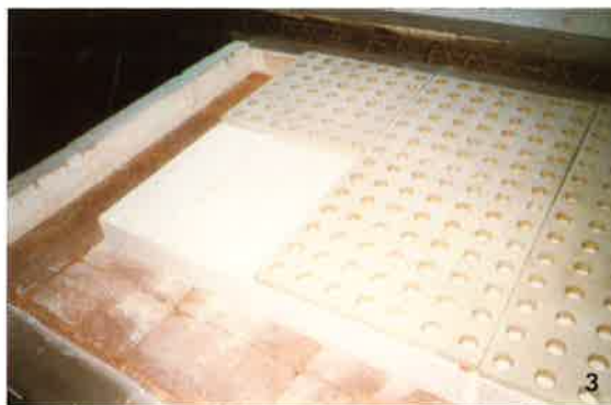
Fig. 3 Innovative kiln car lining with microporous Intoval VL 1000 HT precasts (white) and refractory plate on top. The bottom layer is made of molar bricks
